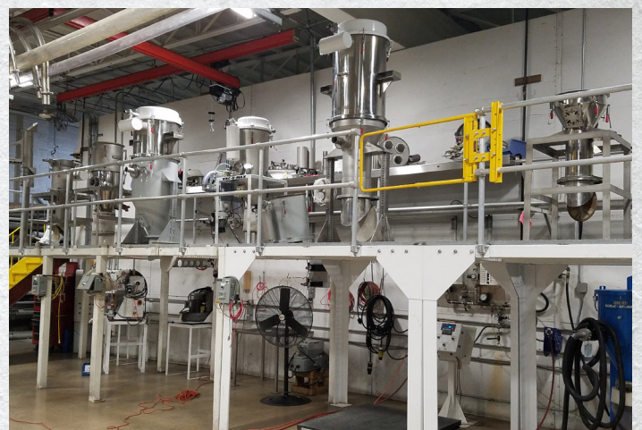
A dedicated test facility, capable of full-scale testing, is used to measure critical material properties including bulk density, flowability, particle attrition, vacuum conveying rates, and vacuum conveyor designs.
