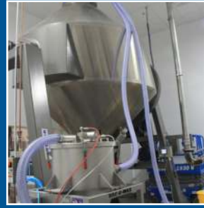
Direct Charge Loading to Mixers/Blenders/Reactors
