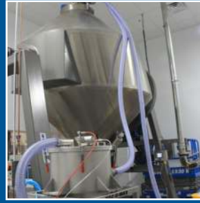
Direct Charge Loading to Mixers & Blenders
