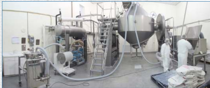
Ingredients are vacuum conveyed from floor-level and directly into tumble blenders without lifting, stair-climbing, and manual dumping of product.
