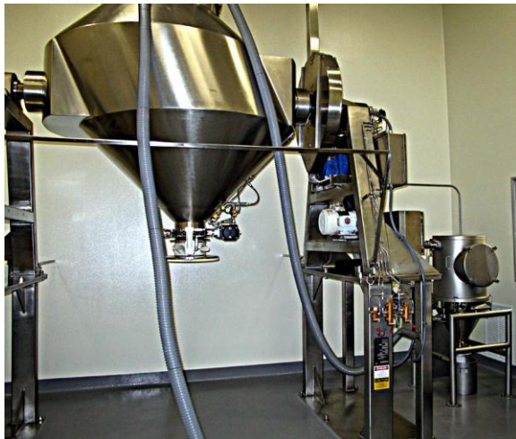
VAC-U-MAX Direct Charge Blender Loading System to a GEMCO Blender. Note the VAC-U-MAX Filter Unit to the right of the blender. System is designed to convey ingredients to the blender from two dump stations.
