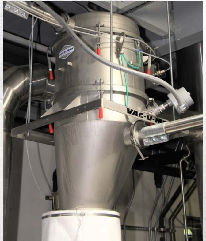
Vacuum system conveys and cleanly discharges 2ft 3 batches of sugar every minute into the mixing tank.
