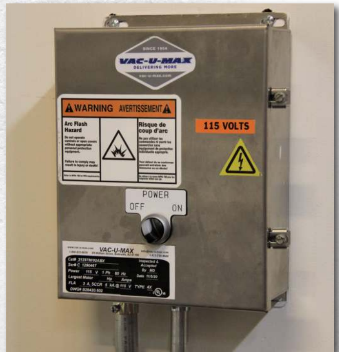
Simple controls start/stop the convey sequence from remote ingredient room.
