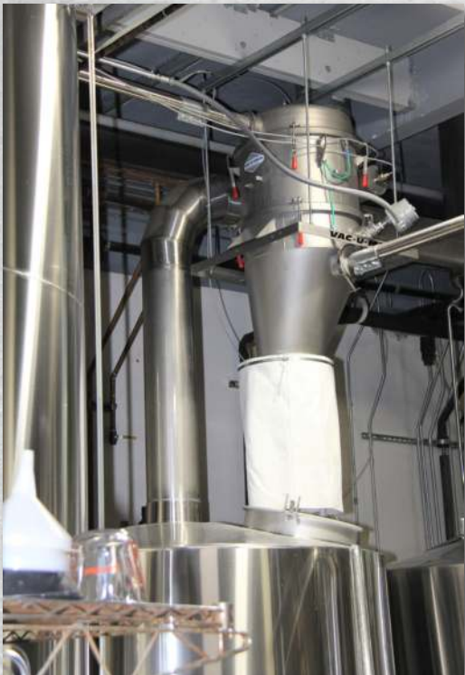
Vacuum conveying system conveys powdered sugar continuously to mixing tank below.
