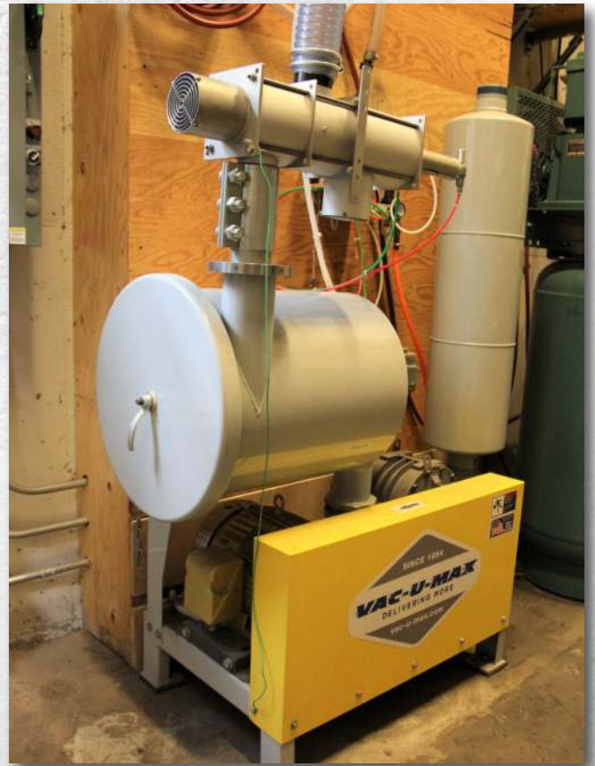
Remote 7.5 HP vacuum pump located in mechanical room.
