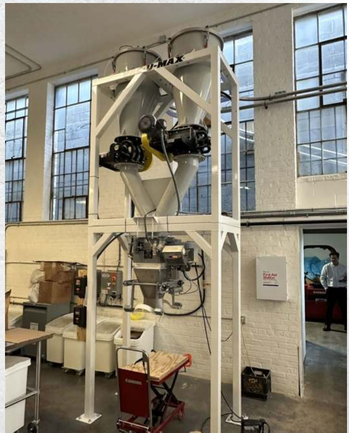
Each cold stone mill has its own vacuum conveyor to deliver the whole grain flour to the bagging station where 25-lb and 50-lb bags are weighed out
