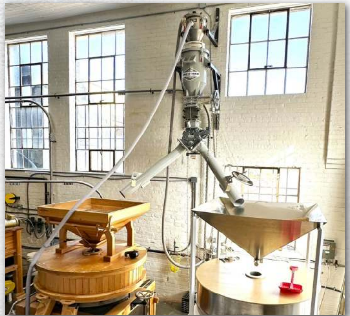
Vacuum conveyor continuously delivers whole grains from bulk bags to two 48”-diameter artisan cold stone mills.
